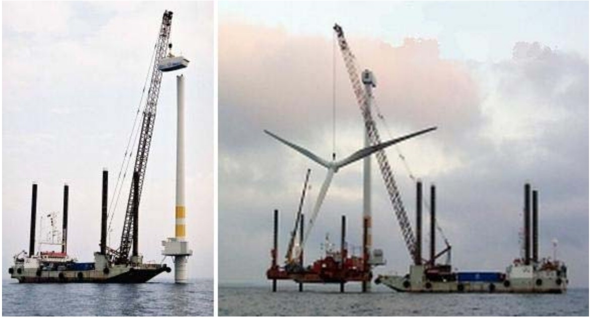
Figure 3-8. The raising of nacelle and rotor by jack-up barge fitted with a crane. Reprinted with permission from: Vestas Wind Systems A/S. Randers, Denmark. 2007. Last accessed March 2007. < http://www.vestas.com/ >
