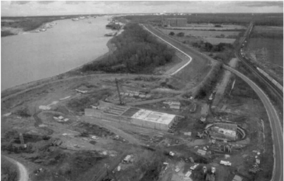
Fig. 3. Construction of the Davis Pond diversion shows the relocated railroad and highway, and the design of the diversion structure. The Mississippi River is flowing towards the top of the photograph to New Orleans.
